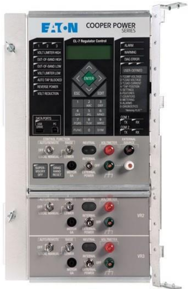
Figure 4. CL-7 multi-phase regulator control.
