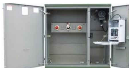
Single-phase pad-mounted regulator with CL-7 control
