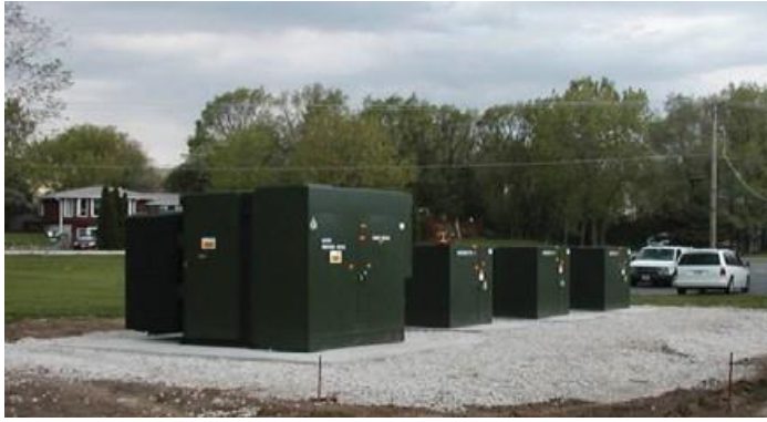
Utility substation placed in the middle of a suburb without the need for fencing and overhead lines
